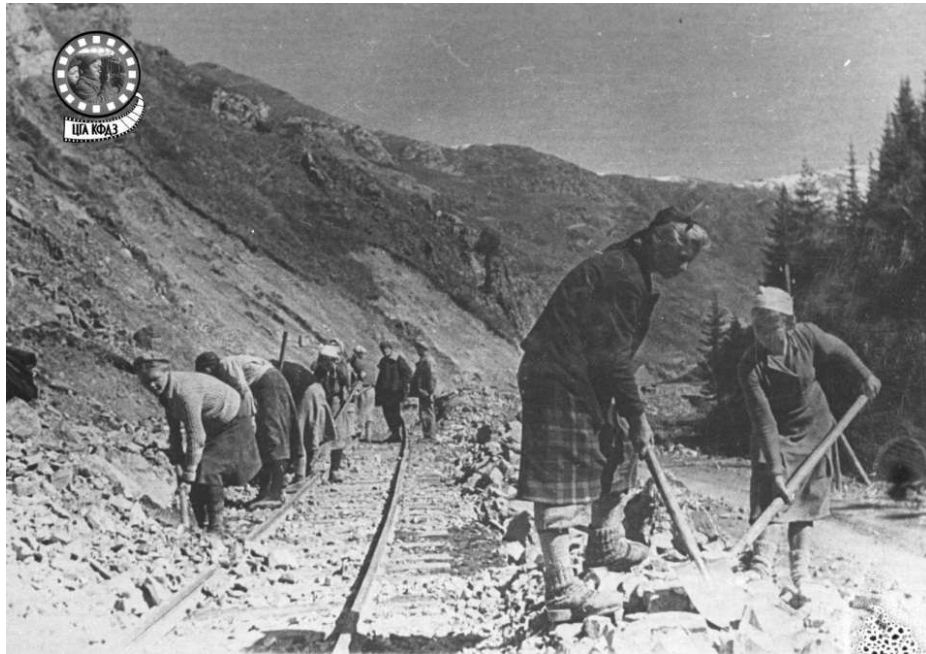
Figure 3. Taldy-Kurgan region. 1944. Tekeli mine. Women construction workers laying a narrow-gauge railway. [TsGA KFDZ RK. 2-37998]
